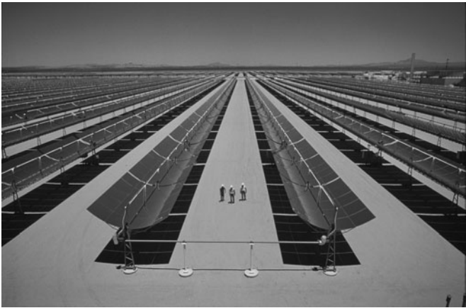
21. Abundant sunshine is one of the most obvious desert resources, and several methods to harness solar power have been developed. This facility in the Mojave desert, southwestern USA, uses sun-tracking mirrors to heat fluid in a pipe, creating steam to drive an electrical generator
